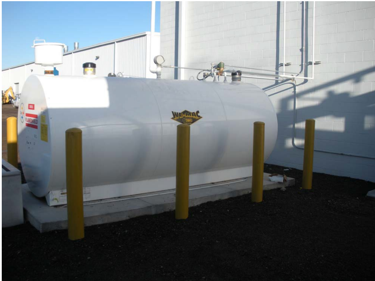
Illustration 73 – Bulk Fuel Storage Tank
