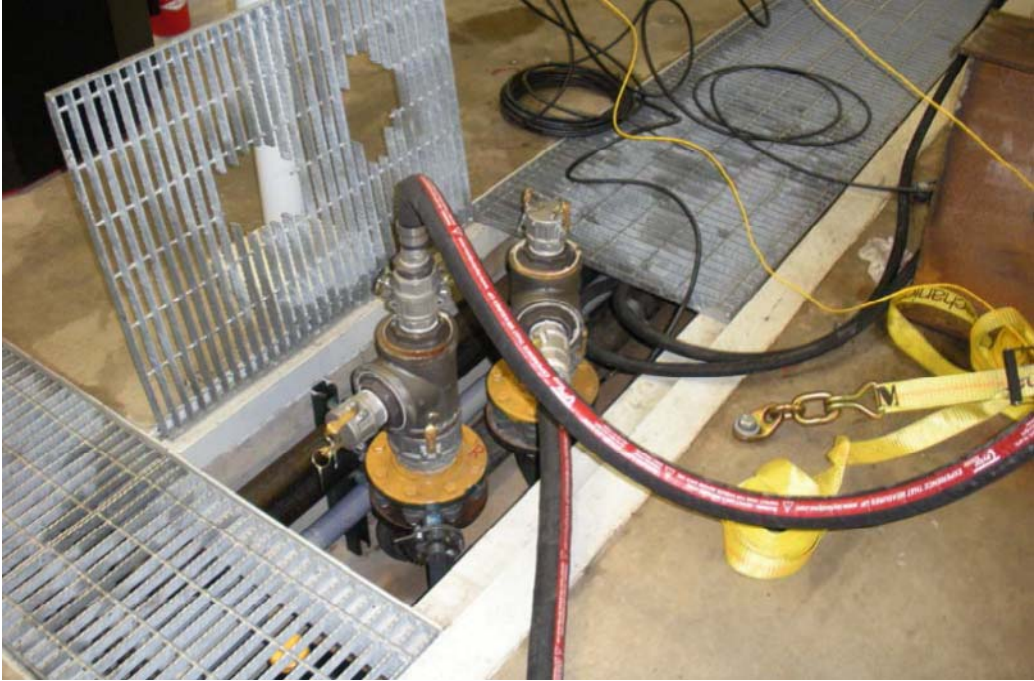
Illustration 89 – Recessed Trench with Cam Lock Water Lines
